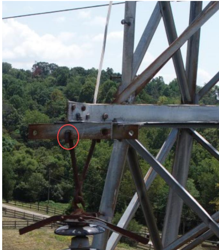
Figure I-8 Structure 2-59: Ovalization of Attachment Hole, Steel Member Rusting, and Hardware Rusting
